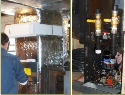
Heat exchange and duct systems resemble conventional equipment
