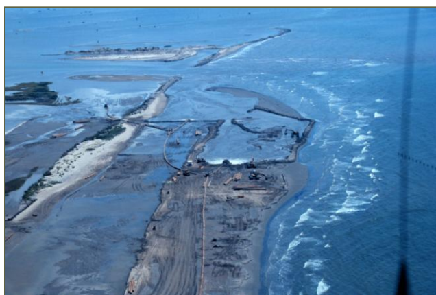
Standard dredging equipment can be readily deployed using proven techniques to build land
