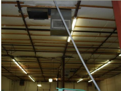
Poorly operating HVAC system to be reconfigured for increased energy efficiency and performance
