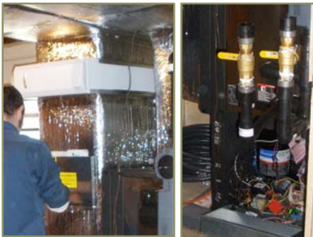
Heat exchange and duct systems resemble conventional equipment
