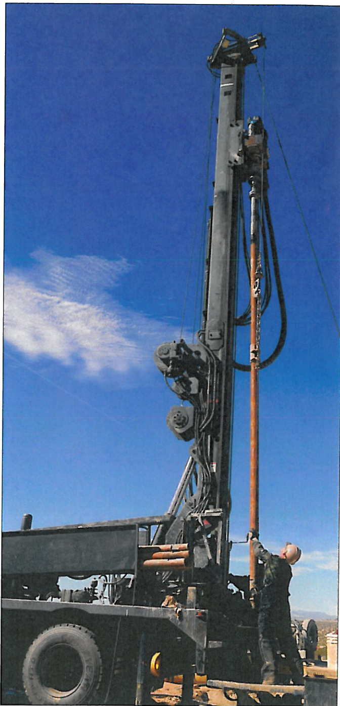
Members of Naval Mobile Construction Battalion 1 drilled three 800- to 1,000-ft-deep holes for the U.S. Navy Geothermal Program Office to support research on local geothermal energy potential at Twentynine Palms, Calif.
